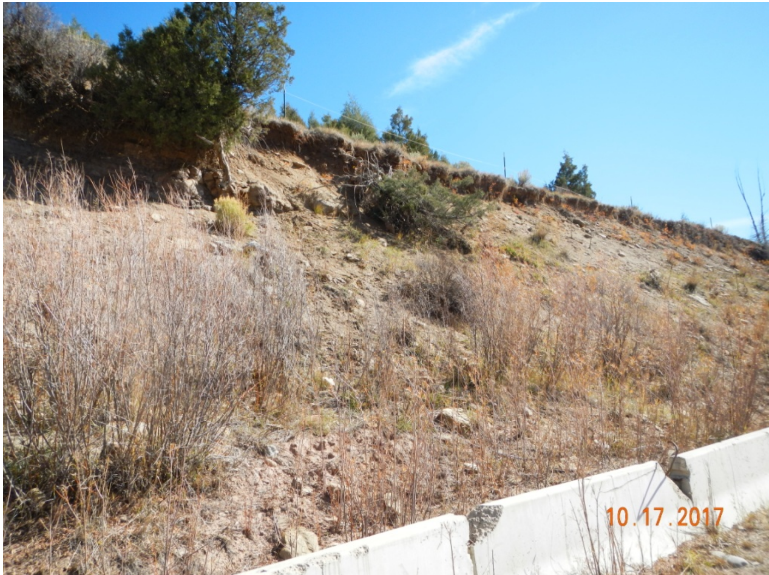
Photo 3. View of the eastern cut-slope. The slope is not stabilized, as evidenced by overhanging vegetation at the top of the slope, and fallen pinyon tree, where eroding soil is exposing roots and resulting in sloughing.
