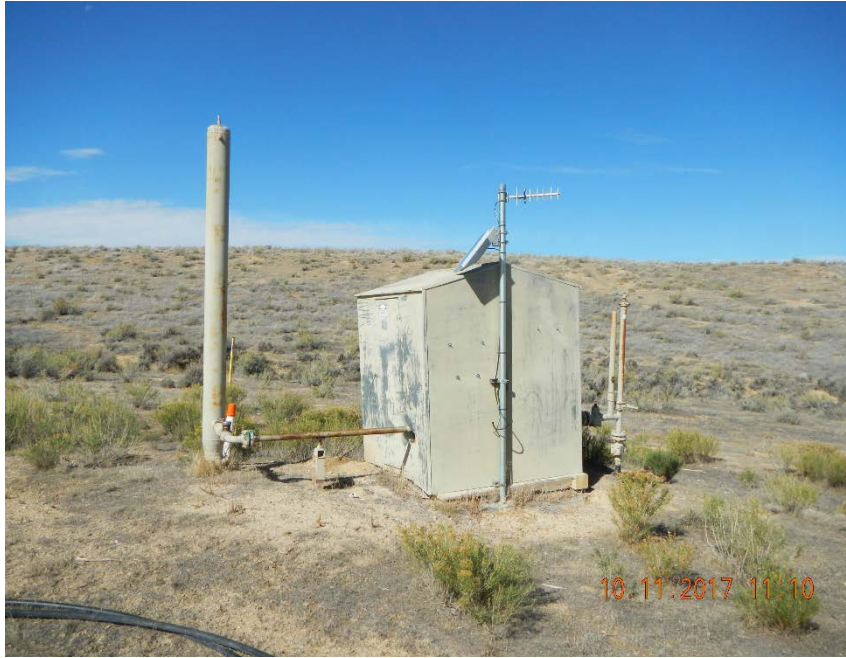
Meter shed and separator looking North
