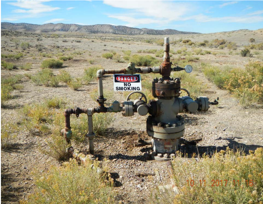
Wellhead looking West
