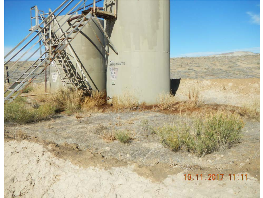
210 bbl condensate tanks with stained soils looking NW
