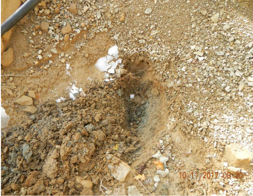
Petro stained soil at outfall into pit
