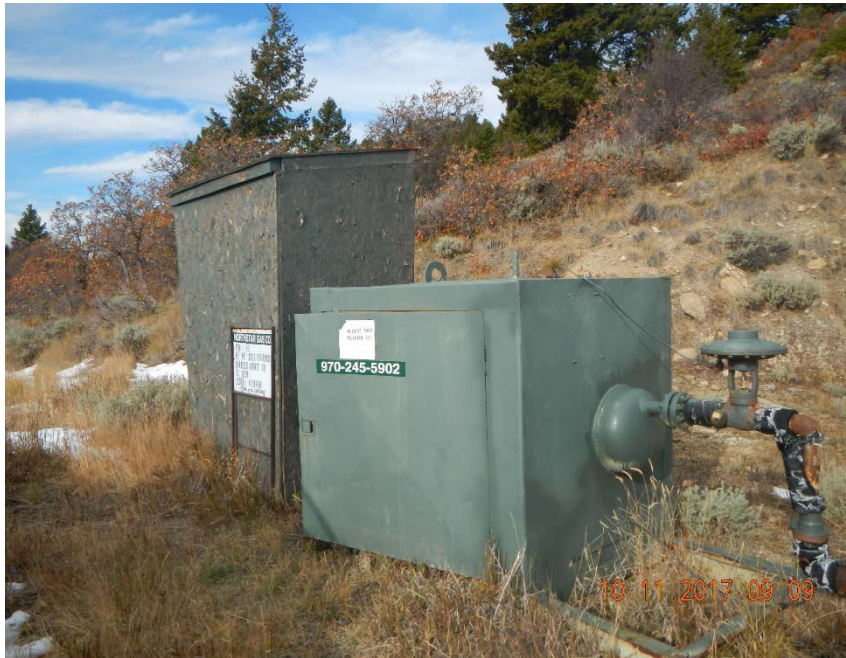
Meter shed and separator looking SW
