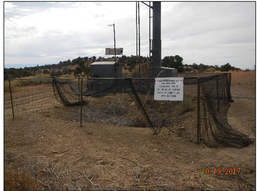
Photo 2. Netting on pit has not been maintained.
