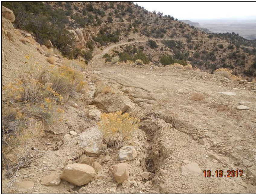
Photo 1. Main road to location has multiple areas of erosion across roadway and sediment migration down gradient of road surface.
