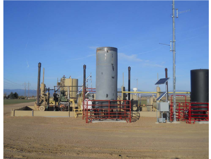
Battery looking west
