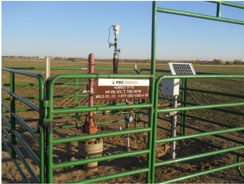
Wellhead looking north
