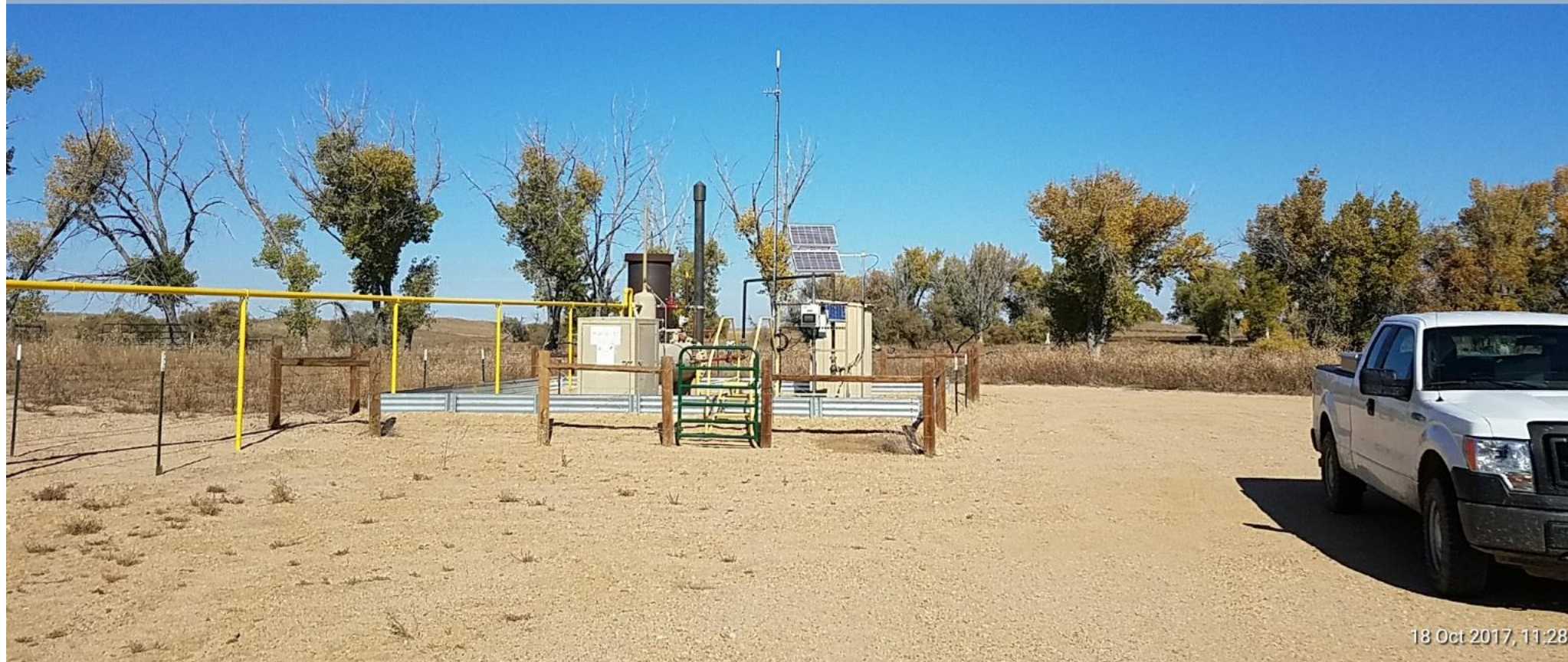
Separator, ECD, GMR Location Number: 330530
