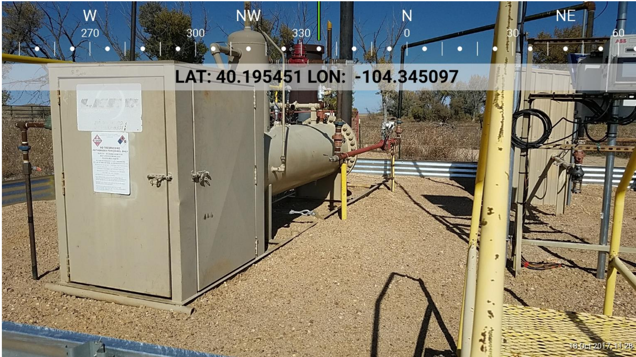
Separator Flood Anchor Location Number: 330530
