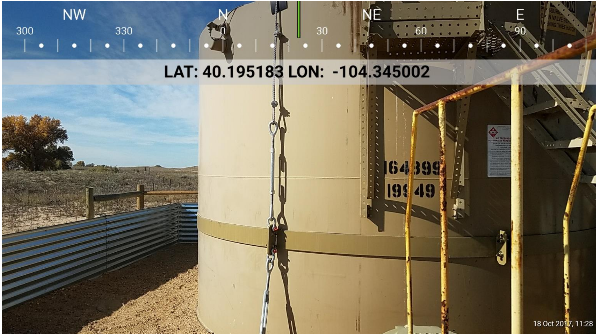
Flood Anchor on Crude Oil Tank
