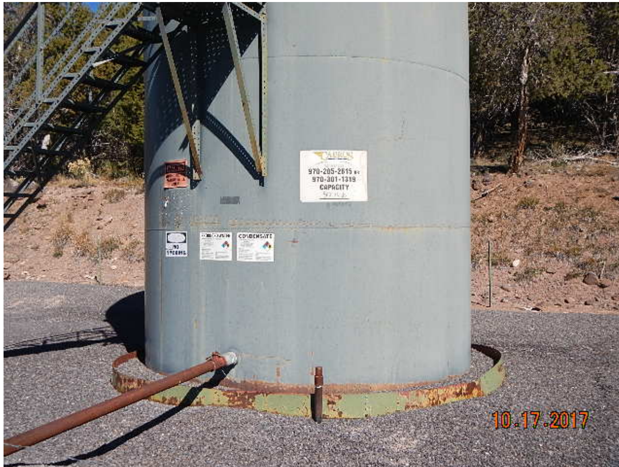
Photo 1. Follow up to inspection Doc#689400114 in response to FIRR Doc#401428489. Capacity has been added to tank. Form 4 has been filed for continued TA status.
