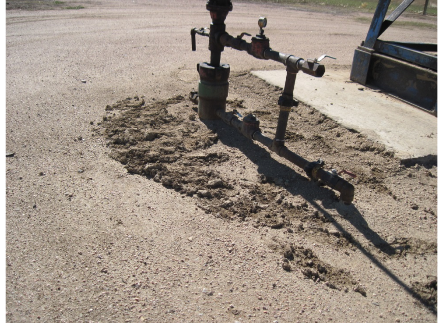
STAINED SOIL CLEANED UP
