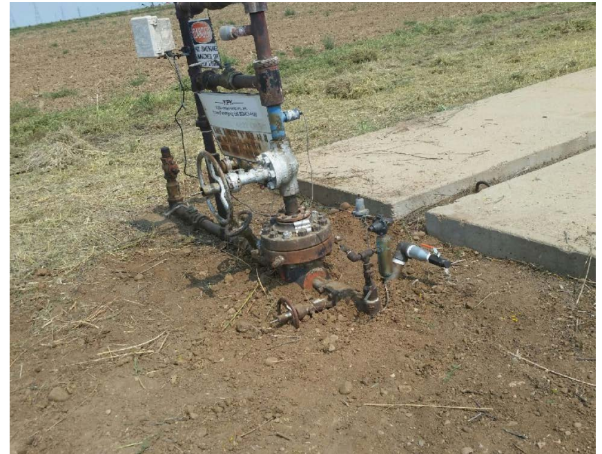
Photo from operator showing bradenhead, weeds controlled.
