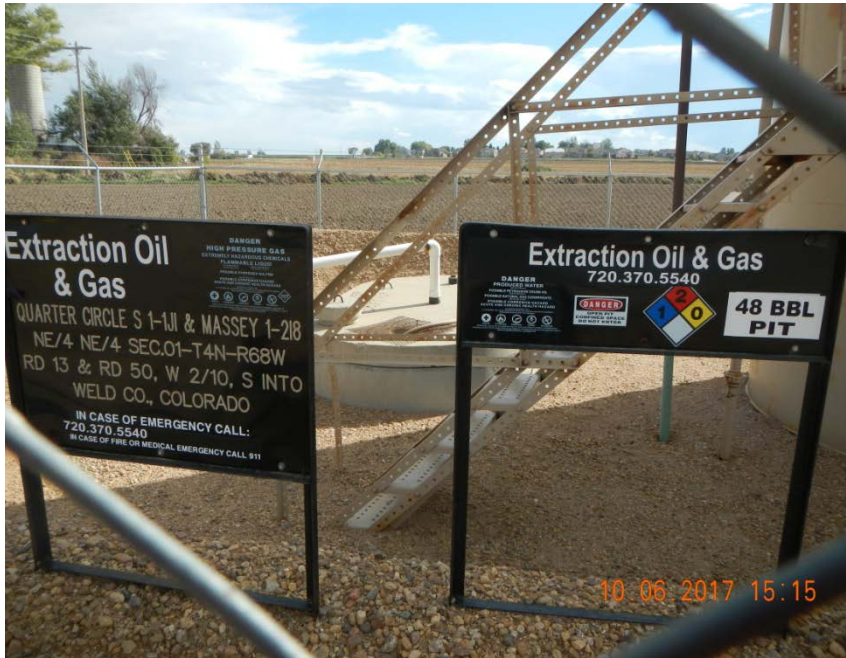
Produced water vault capacity placard
