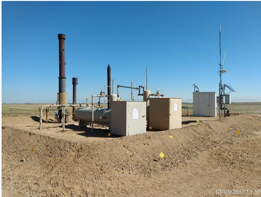
Separators, ECD, meter run, & ancillary equipment.
