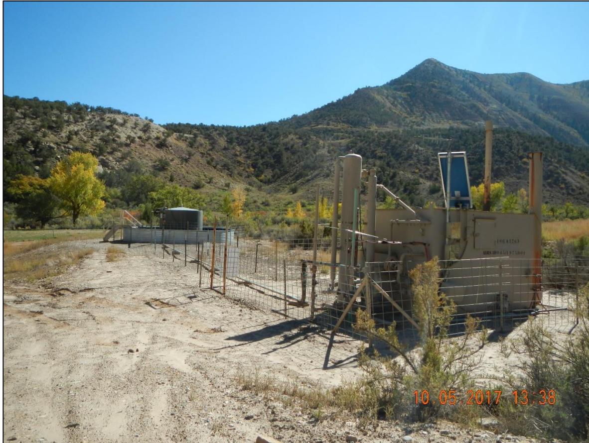
Tank battery and separators
