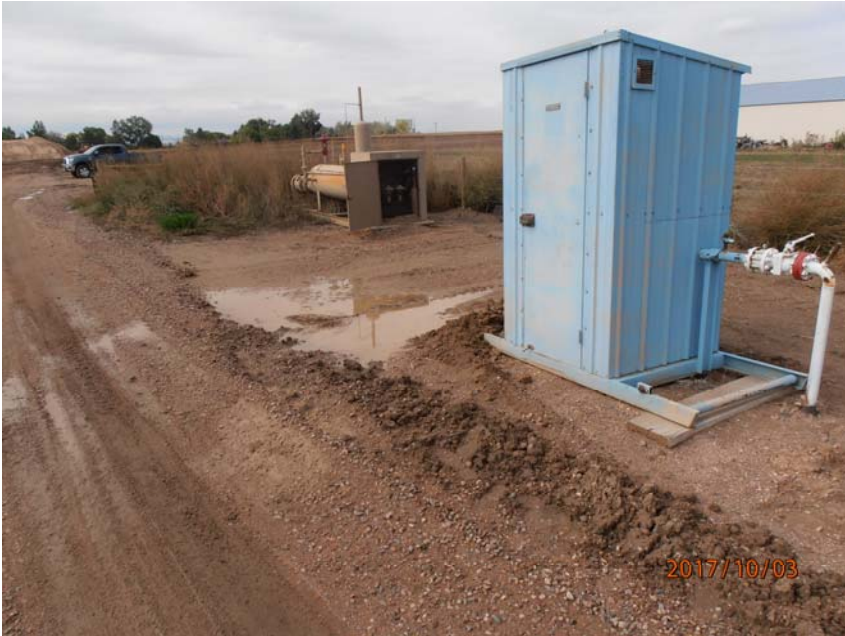
Photo 5: Separator and meter shed on north side of location.
