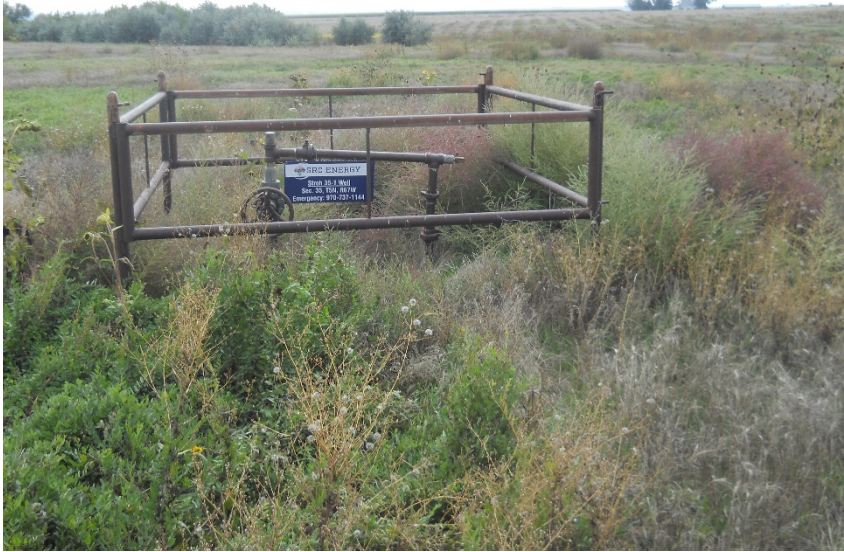
Wellhead looking south. Wellhead sign is reading the Stroh 35-1, well is the Stroh 35-2. Actively growing weeds at wellhead need to be controlled
