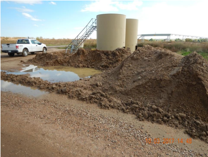
Photo 5. Photo taken from the western battery location, facing Southeast. Did not observe any stormwater BMPs during the removal of equipment.
