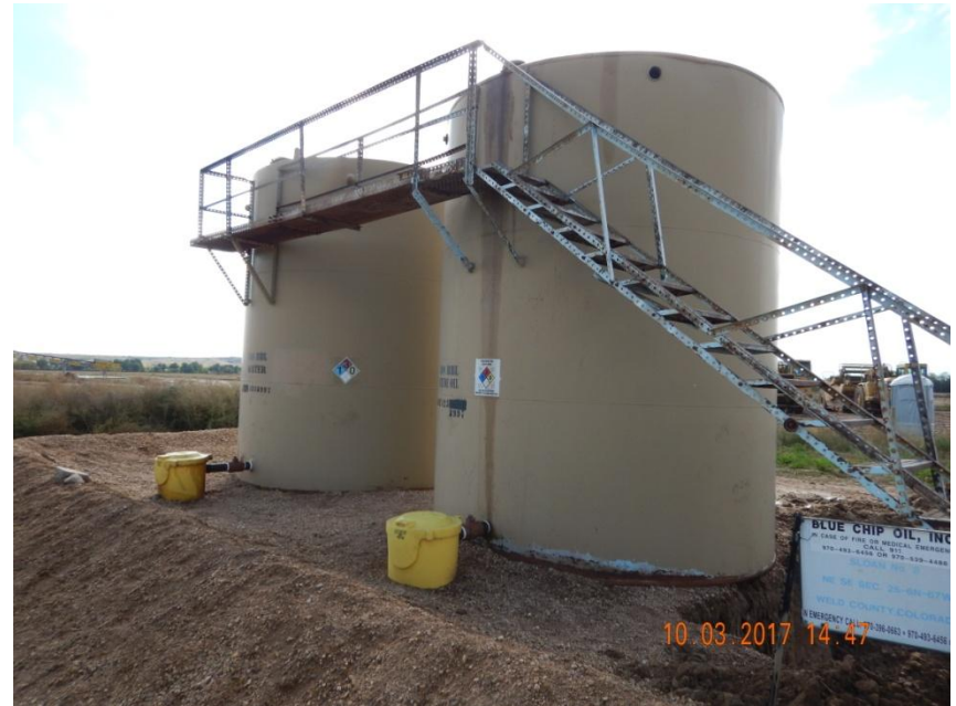
Photo 2. Photo taken from the battery location, facing South. Equipment still at location needs to be removed per Rule 1004.a.
