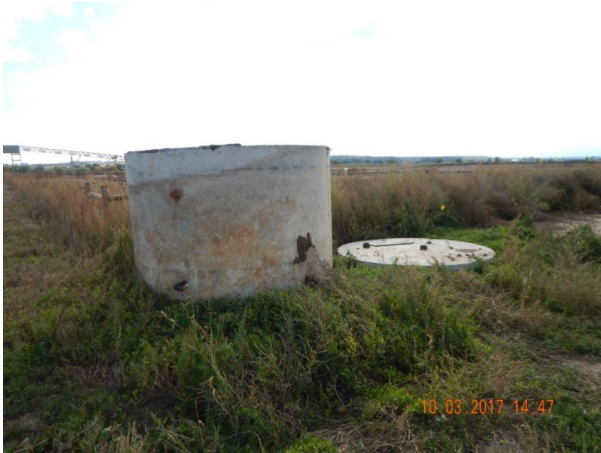
Photo 3. Photo taken from the battery location, facing Southeast. Equipment still at location needs to be removed per Rule 1004.a.
