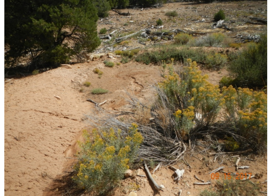
Photo 4: View of silt trap in the northeastern portion of the project area that is nearly full of sediment and will soon require maintenance.
