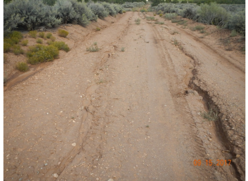
Photo 6: View of more erosional channels up to 12 inches deep, along the access road.
