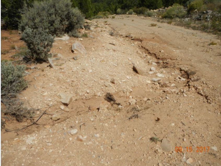
Photo 5: View of erosional channel approximately 18 inches wide and 10 inches deep, along the access road.
