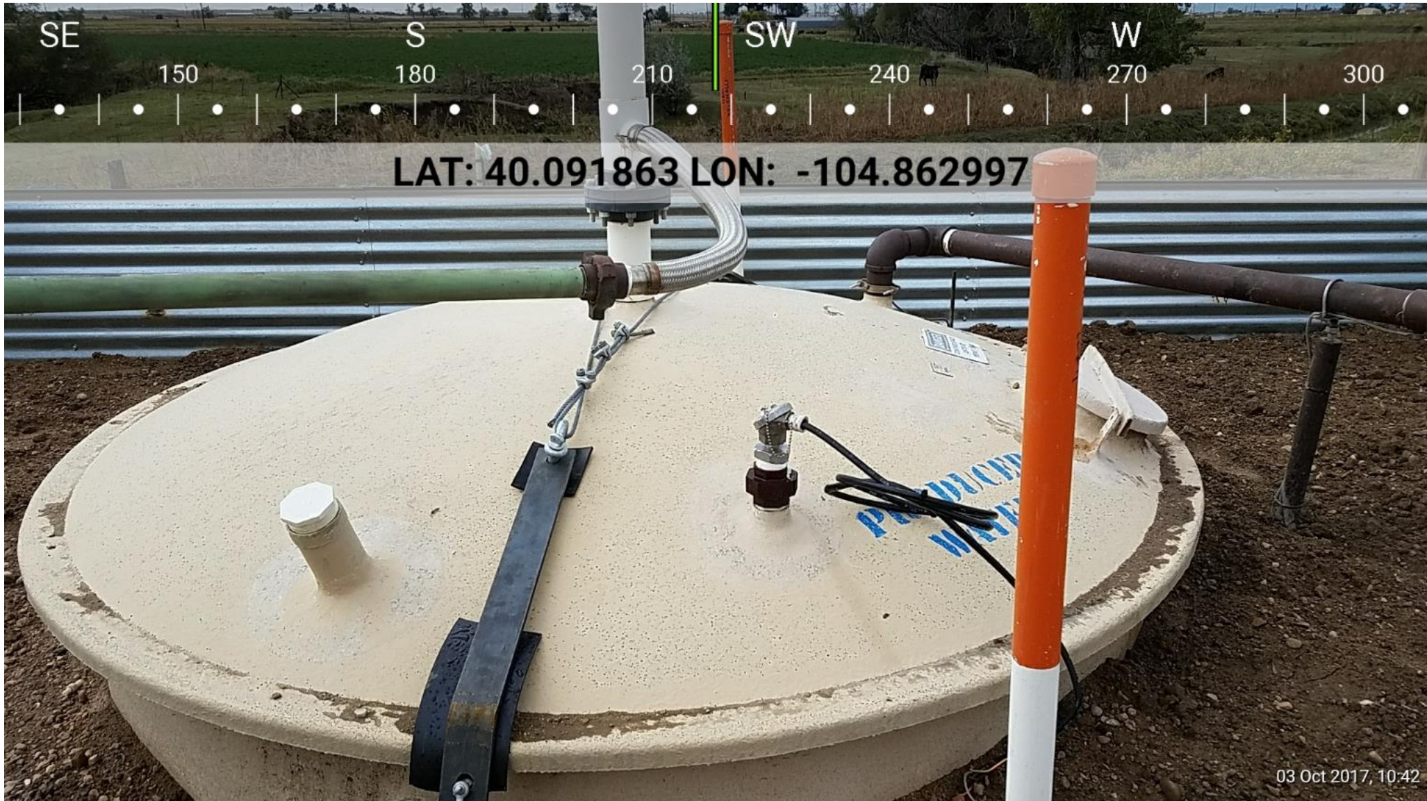
Flood Anchor on Produced Water Tank
