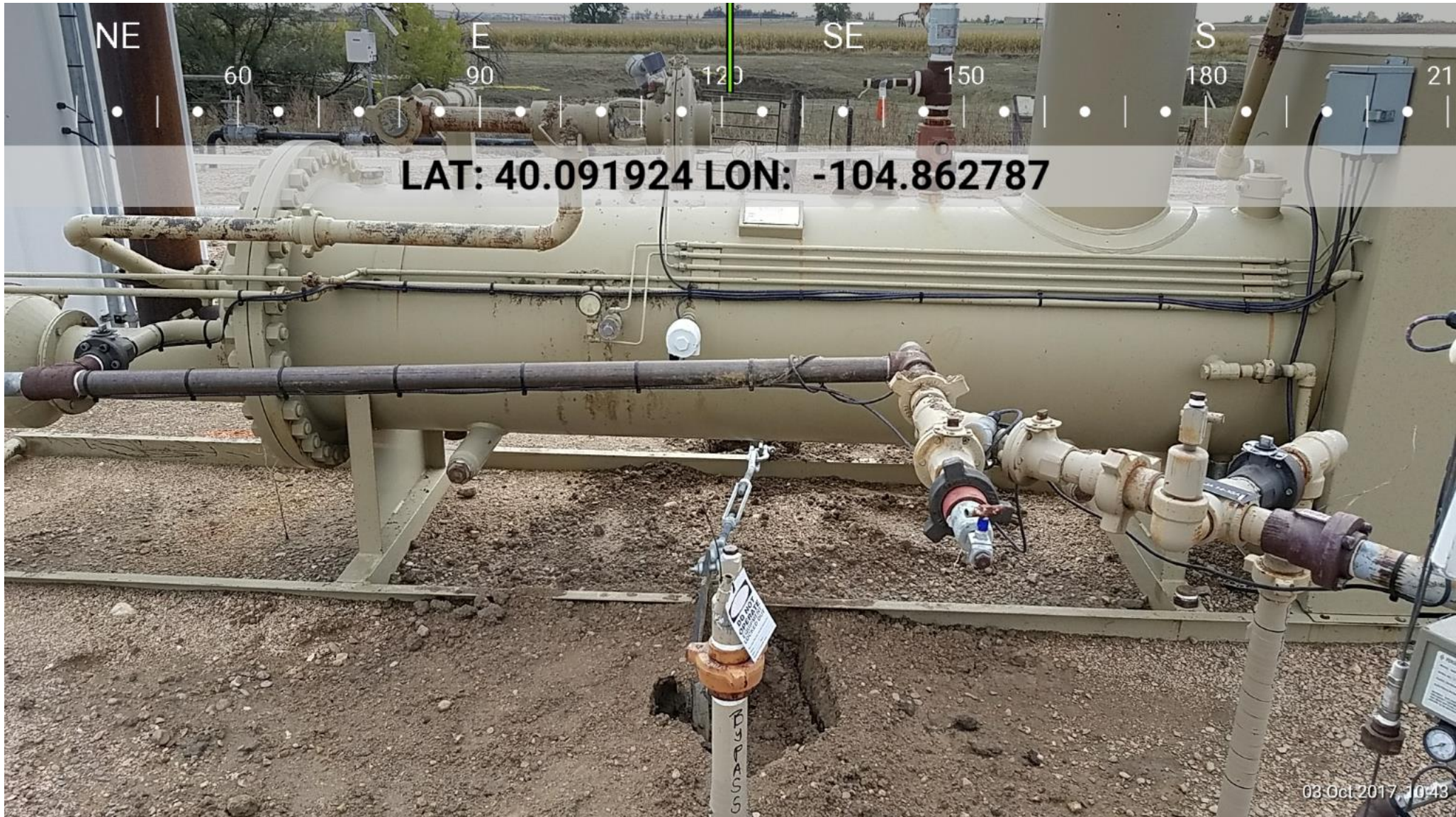
Flood Restraint on Separator Location Number: 311459
