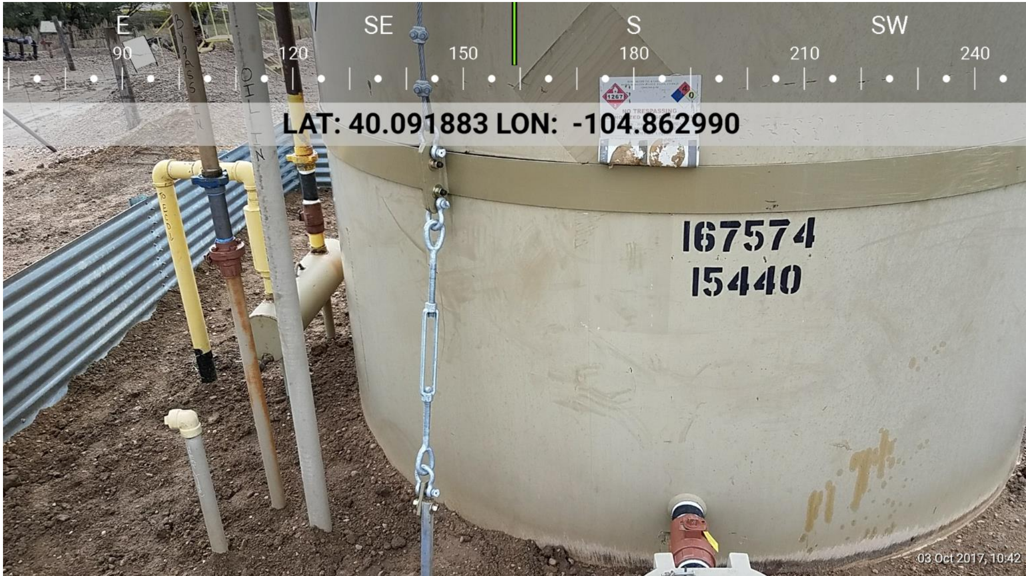
Flood Anchor on Crude Oil Tank
