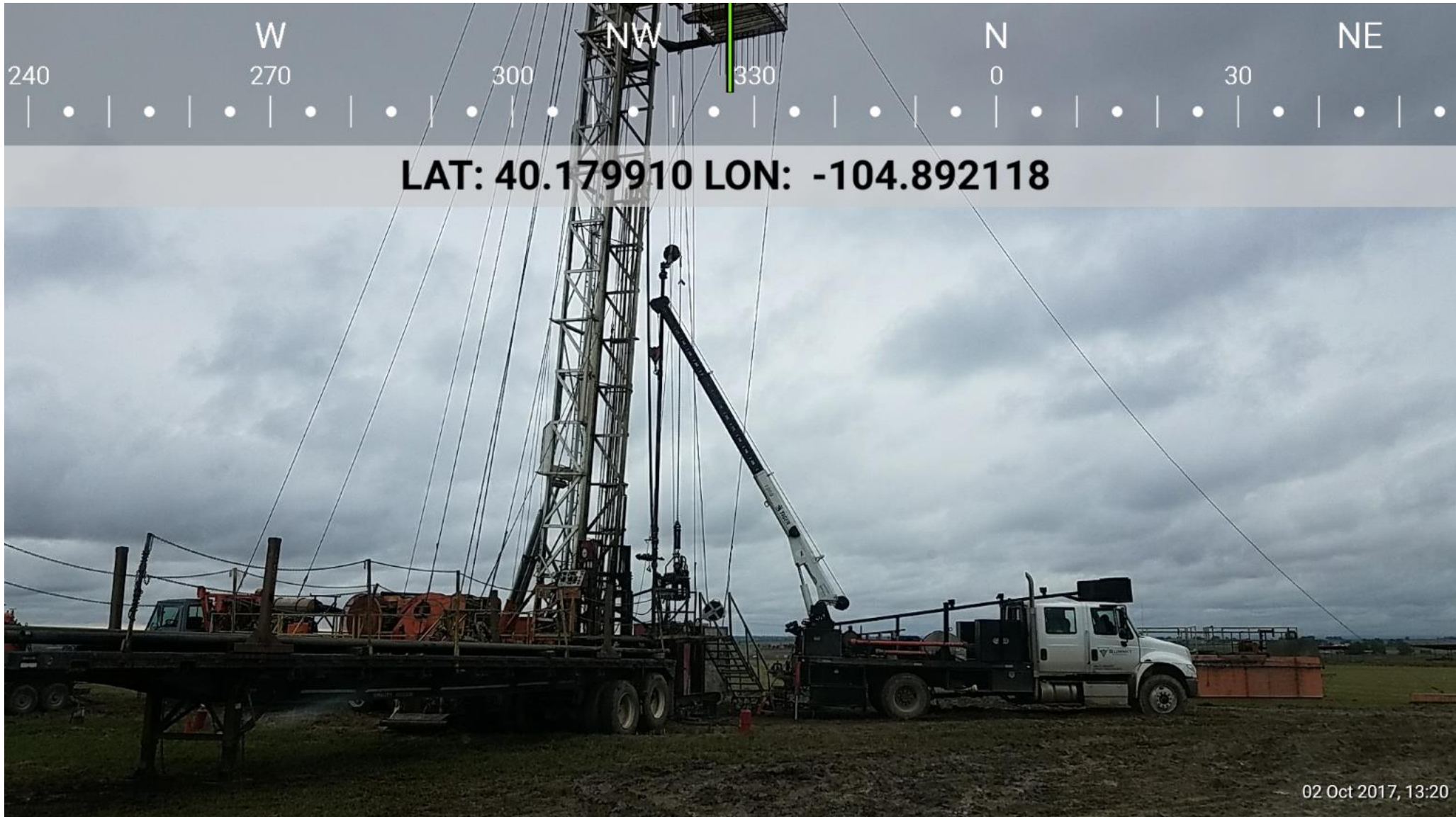
Slick Line Unit and Basic 1652 Rig Location Number: 330225
