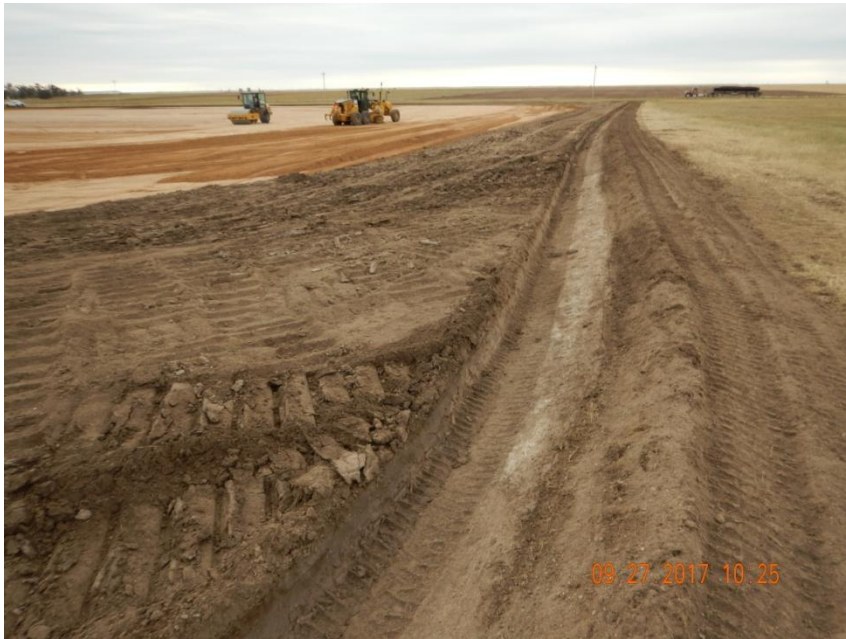
Photo 5. Photo taken from the northwest location, facing South. Temporary BMP's (ditch and berm) have been installed.
