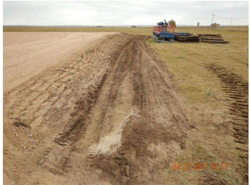
Photo 2. Photo taken from the southeastern location, facing East. Temporary BMP's (ditch and berm) have been installed.
