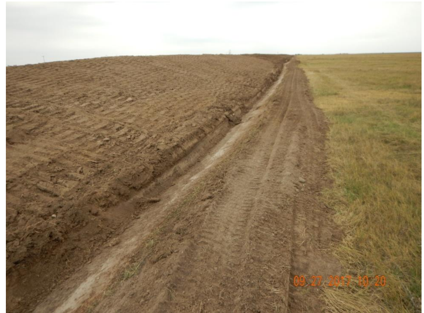
Photo 4. Photo taken from the northeastern location, facing West. Temporary BMP's (ditch and berm) have been installed. Appears topsoil has been temporarily stabilized and stored along the northern location.
