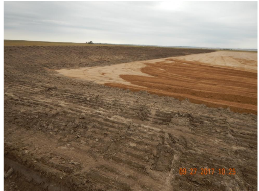
Photo 6. Photo taken from the northwest location, facing East. Appears topsoil stockpile has been temporarily stabilized as well as cut slope areas.
