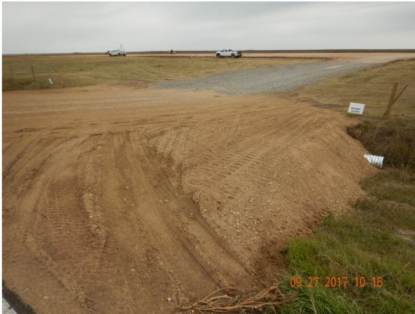
Photo 1. Photo taken from the entrance of location, facing Northwest. Tracking pad devices have been installed at the entrance.
