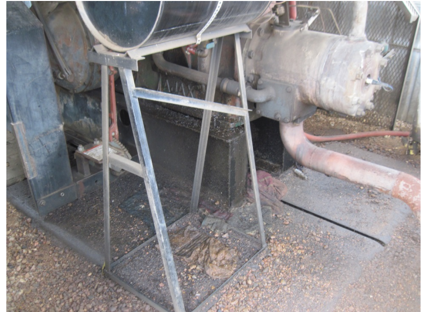
SOILED DIRT INSIDE PUMP JACK HOUSE AT MOTOR MOUNTS
