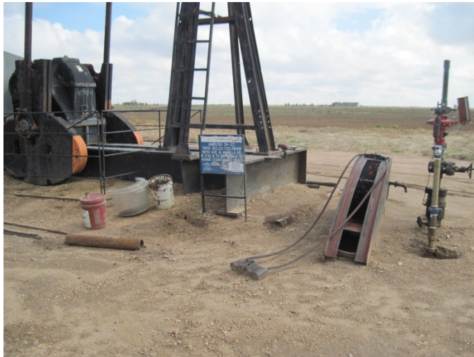
WELLHEAD SIGN AND UNUSED PIPE, EQUIPMENT RODS, PIPE TBG ANCHOR
