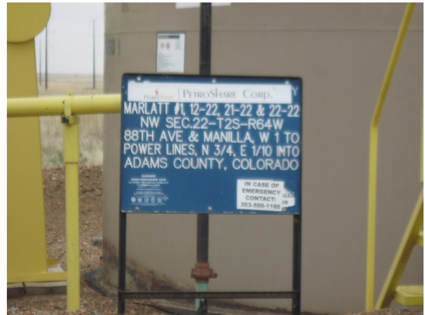
MARLATT TANK BATTERY
