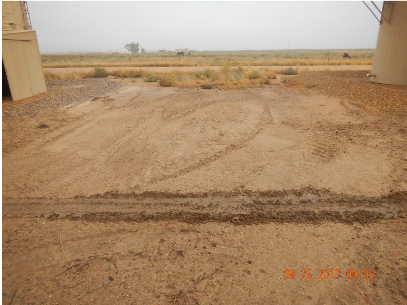
Photo 1: Photo taken from the tank battery facility. Photo shows the seven (7) pipe risers identified in the previous inspections have been removed.
