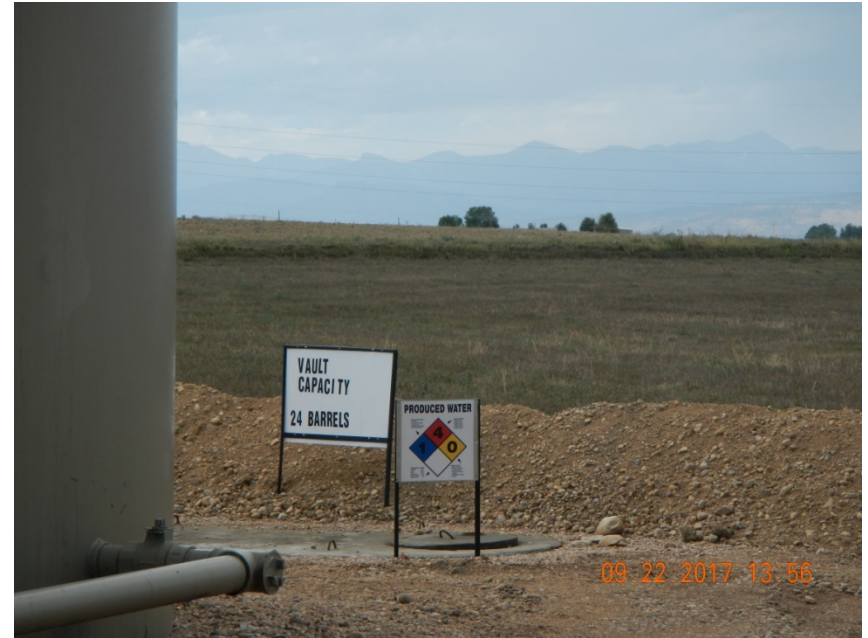
Produced water vault placard on 9/22/17
