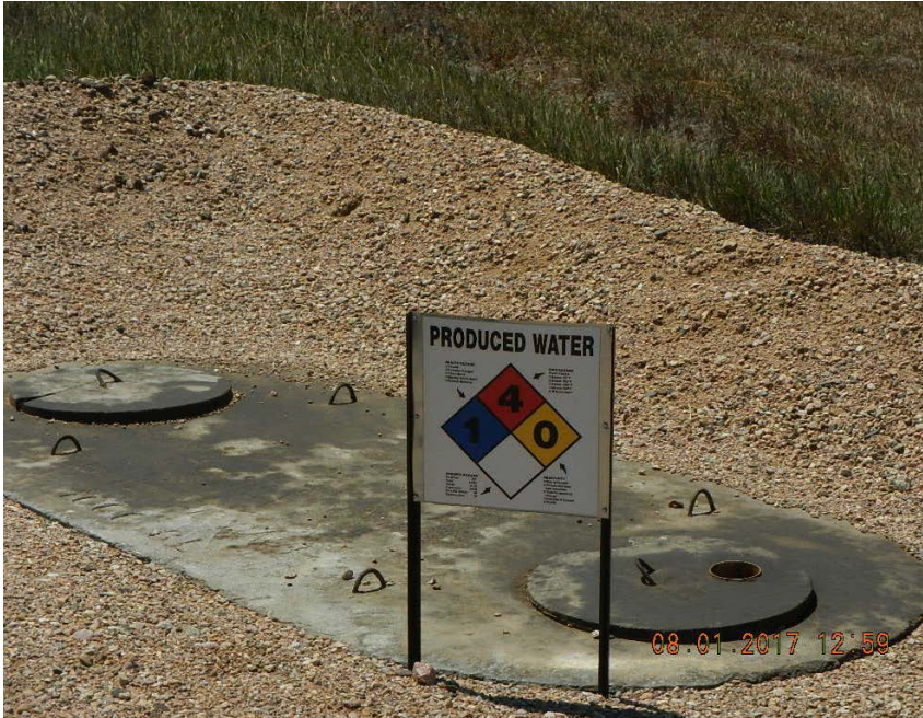
Produced water vault placard on 8/1/17
