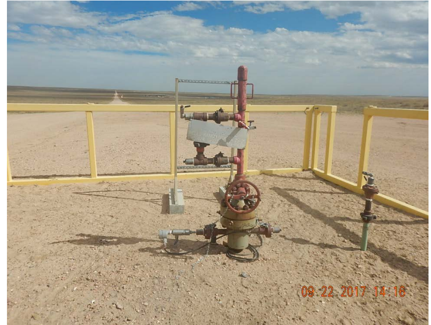
Photo 2: Wellhead sign is faded. Well is TA, looking E.
