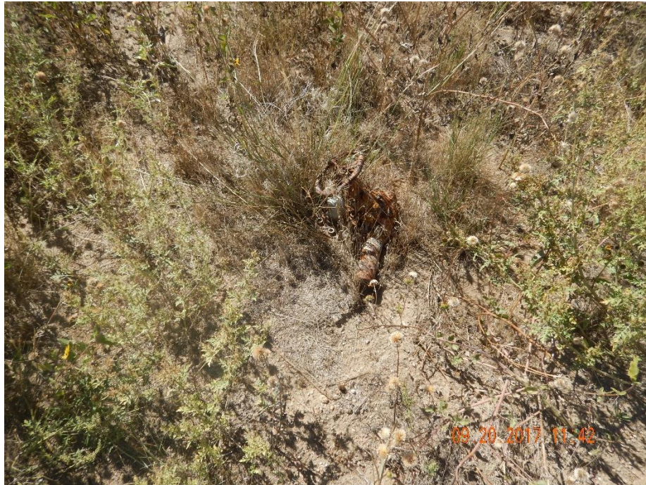
Photo 1: Photo taken from the well location. Photo shows pipe equipment has not been removed per corrective actions and reclamation requirements.
