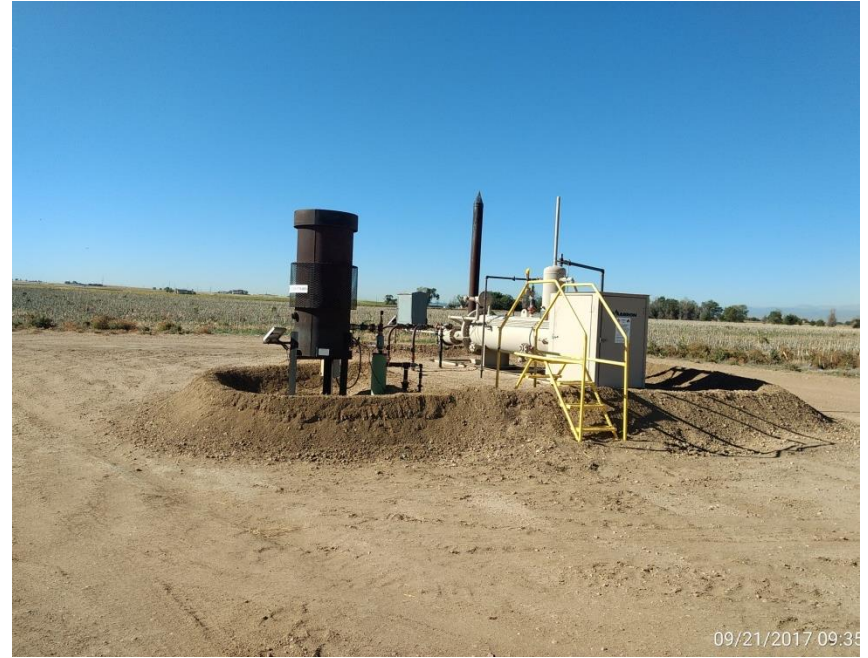
Separator, ECD, and meter run
