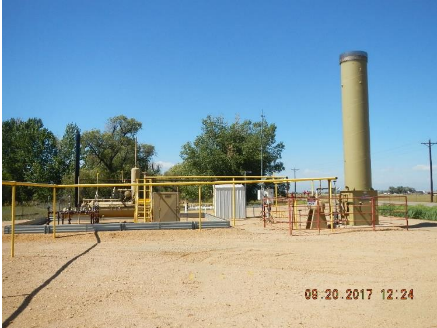
Separator, ECD, GMR, Pig from east Location Number: 336259
