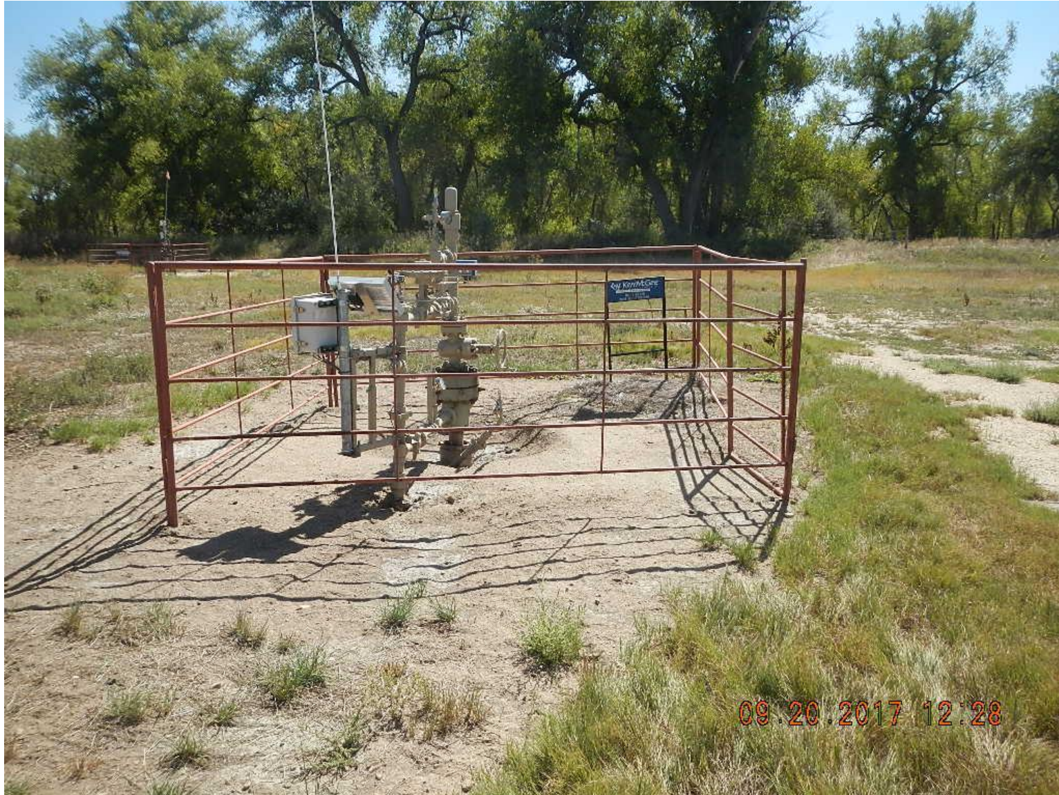
Wellhead Fort 41-36 Location Number: 336259
