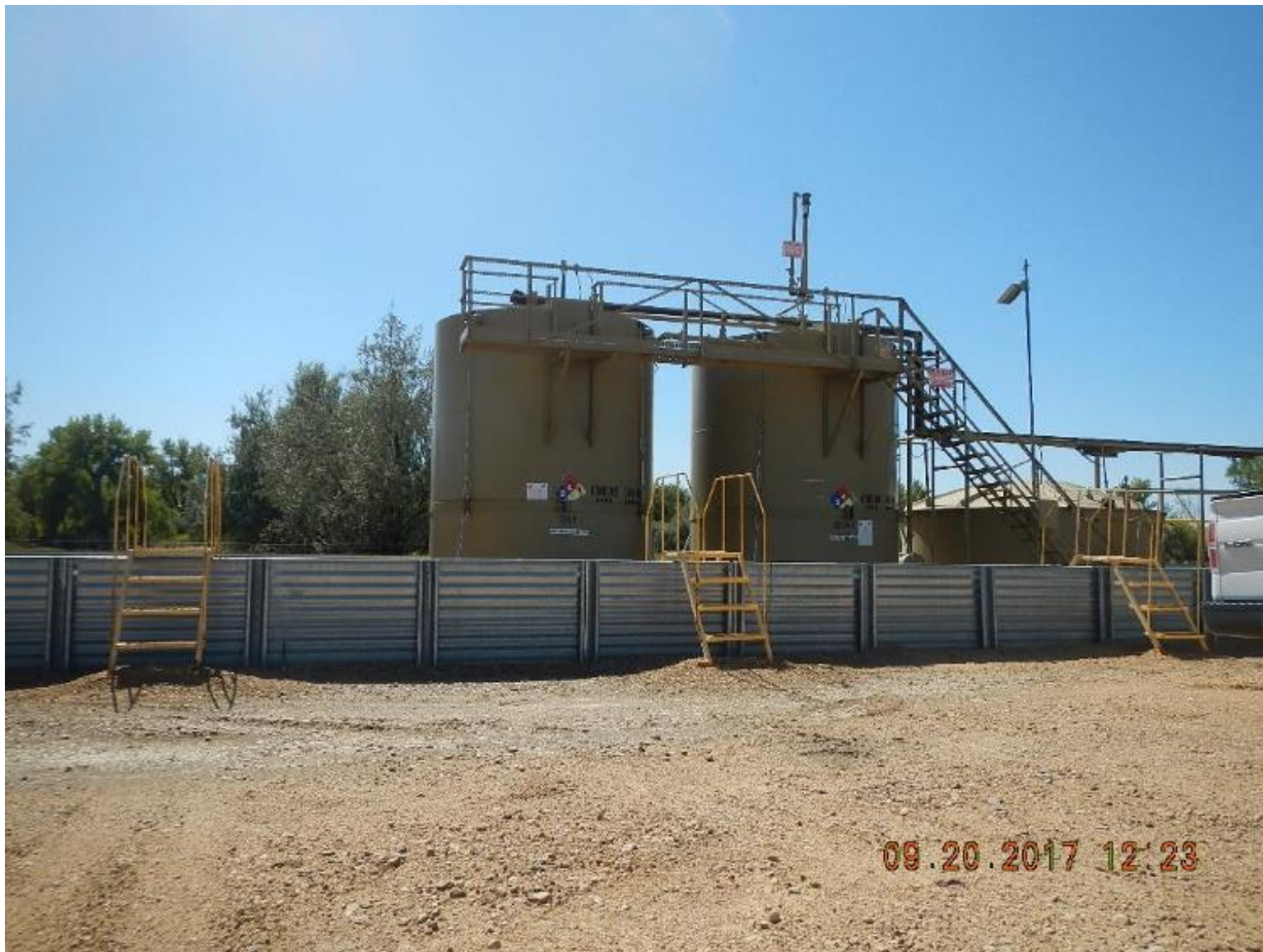
Battery from north Location Number: 336259
