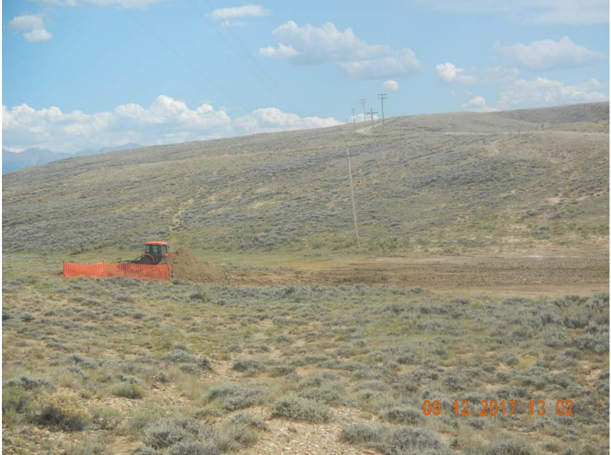
Spill area from upgrade
