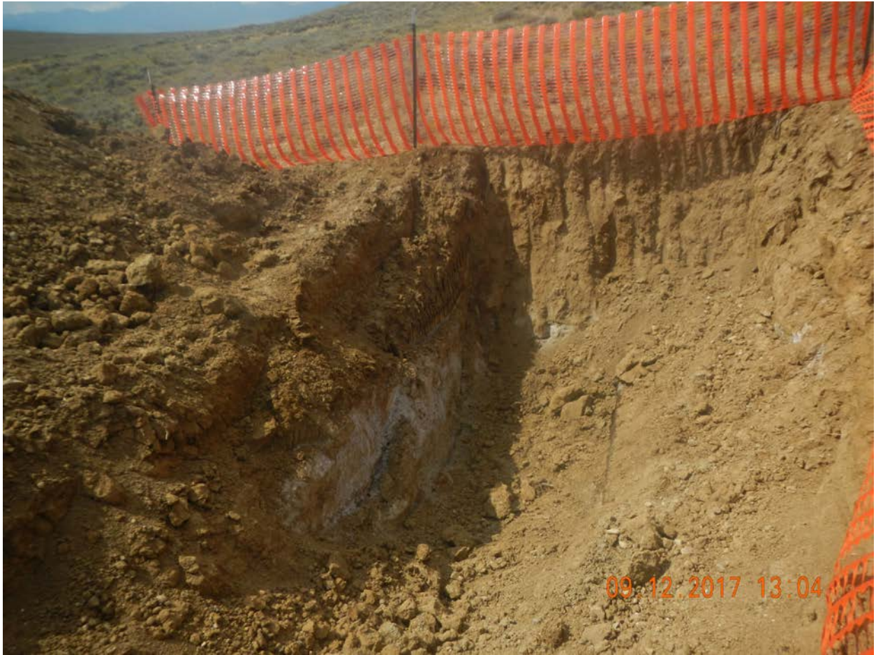
Flowline, repair is observable
