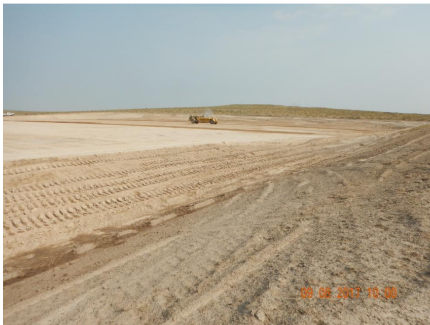
Photo 1. Photo taken from the southern location, facing Northeast. Construction operations still underway. South and west fill slopes appear to be temporarily stabilized even though equipment has not properly tracked perpendicular to the slope. Water truck at location mitigating fugitive dust from operations.
