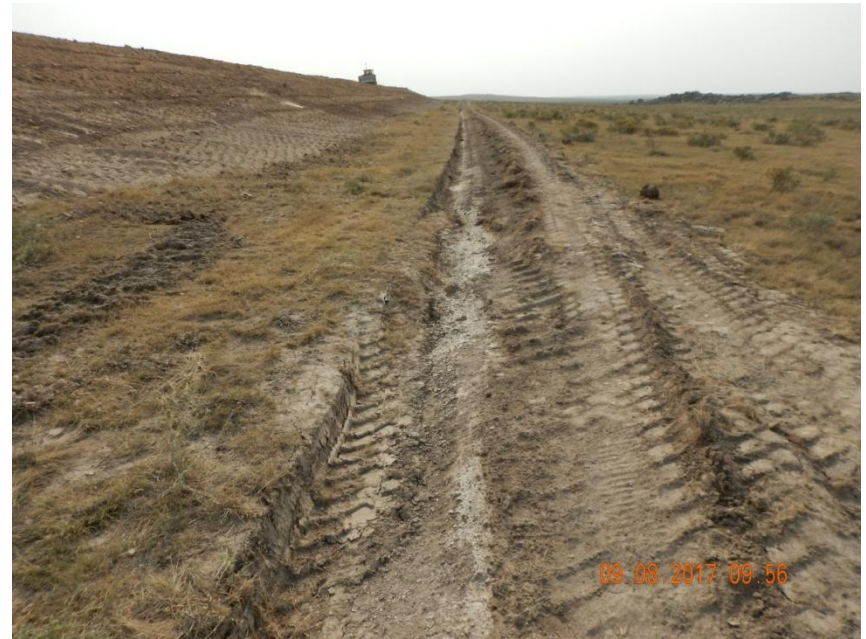
Photo 4. Photo taken from the western location, facing South. Temporary BMP (i.e., ditch) installed around in the entire perimeter of the location.
