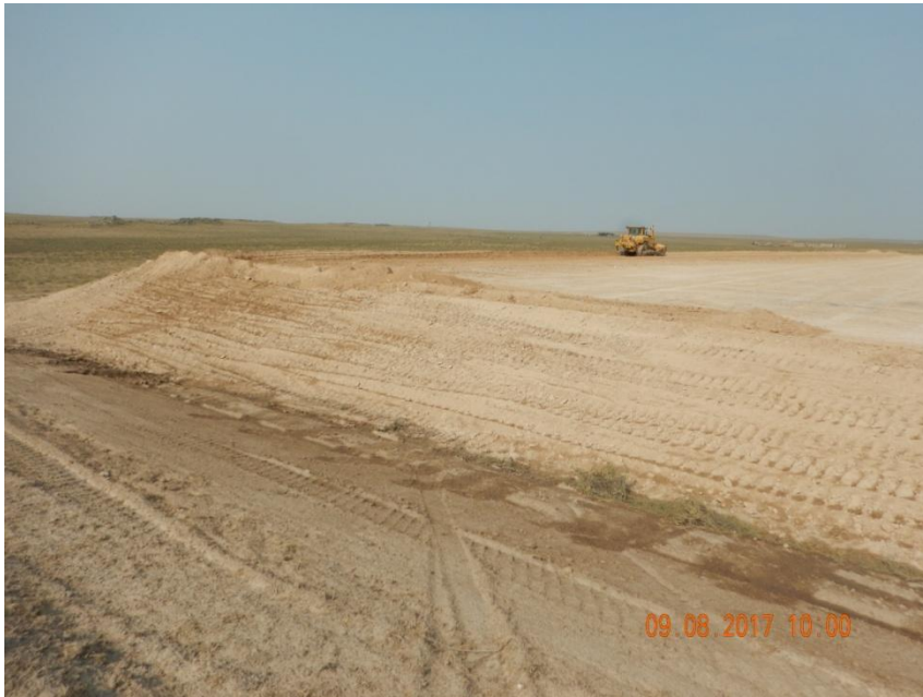
Photo 3. Photo taken from the southern location, facing Northwest. Construction operations still underway. South and west fill slopes appear to be temporarily stabilized even though equipment has not properly tracked perpendicular to the slope.
