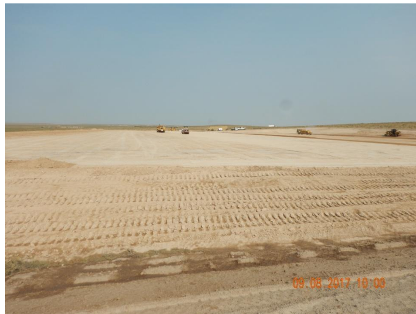
Photo 2. Photo taken from the southern location, facing North. Construction operations still underway. South and west fill slopes appear to be temporarily stabilized even though equipment has not properly tracked perpendicular to the slope.
