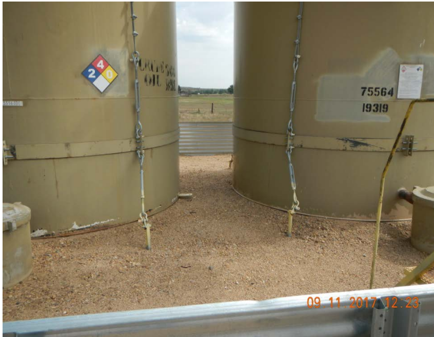
Crude oil tank anchors
