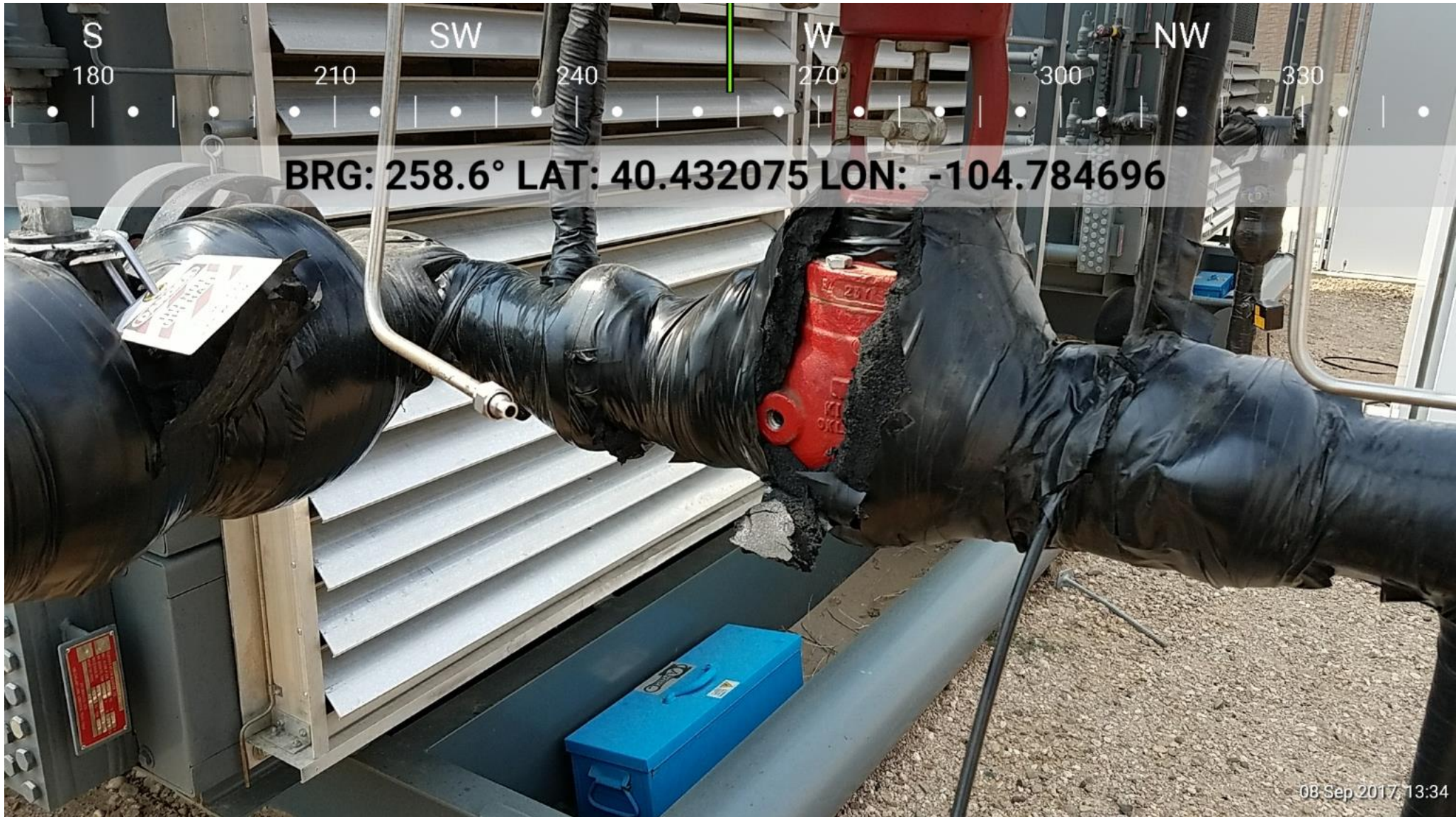
Threaded outlet on compressor outlet where nipple failed.
