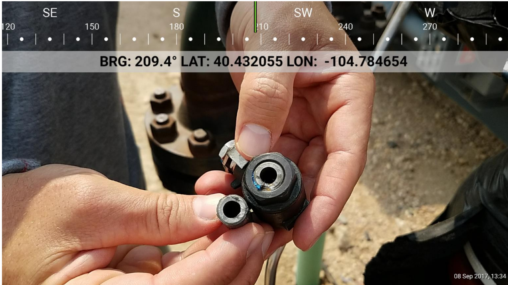
Close view of failed nipple. Location Number: 434391
