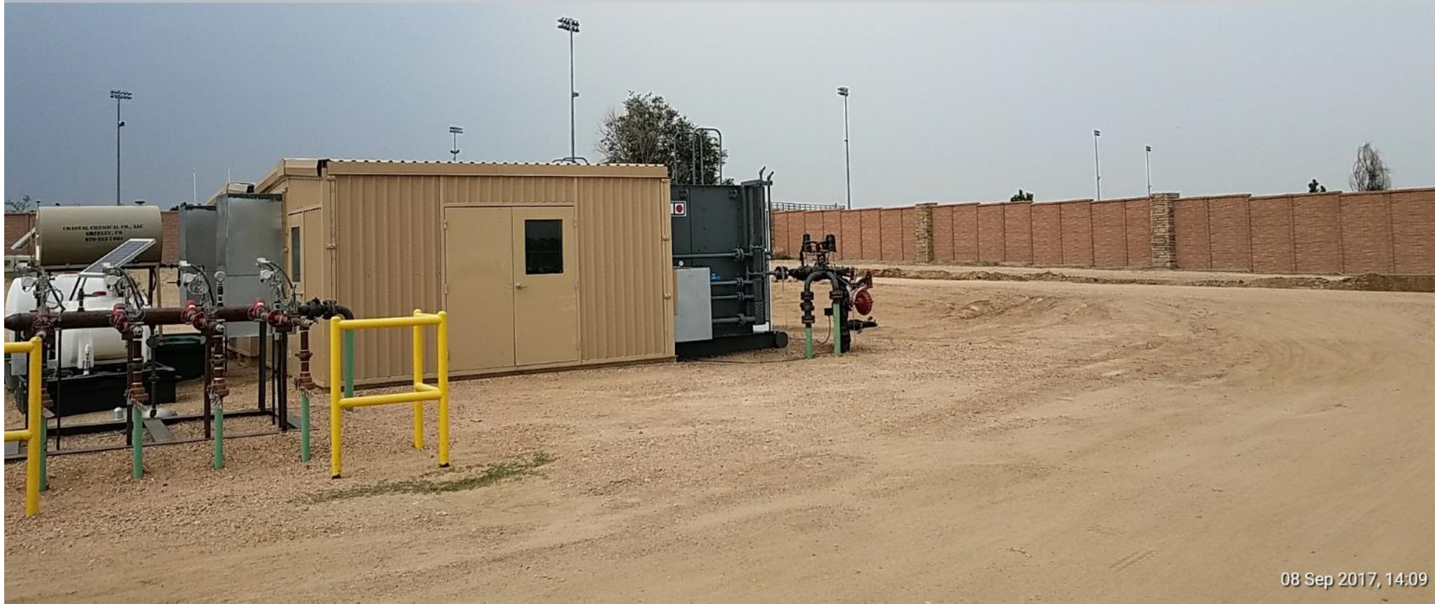
Compressor installation where part failure occurred.
