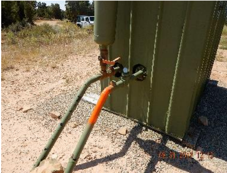
Photo 3: Flowline riser at meter house open to atmosphere.
