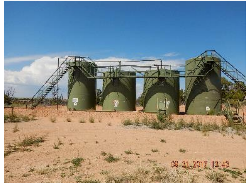
Photo 12: Production tank battery.
