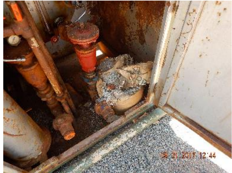
Photo 8: Deteriorated bag of material inside separator box.
