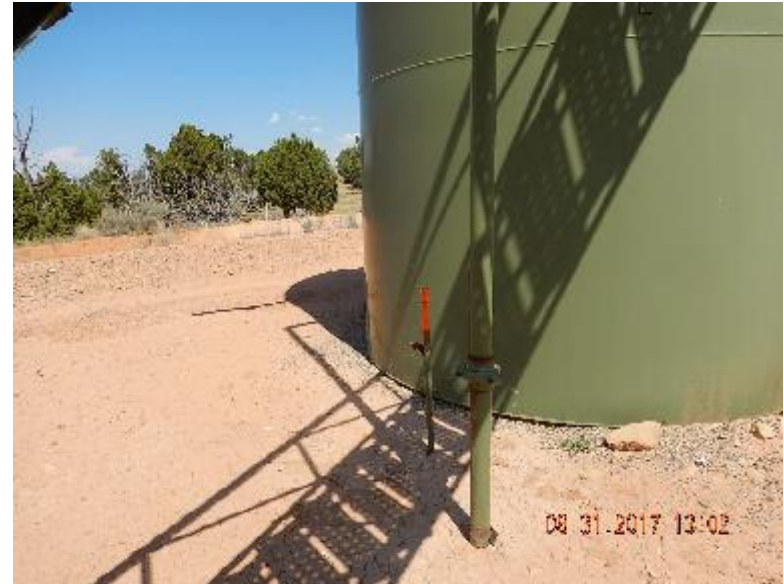
Photo 6: Riser in production tank battery.
