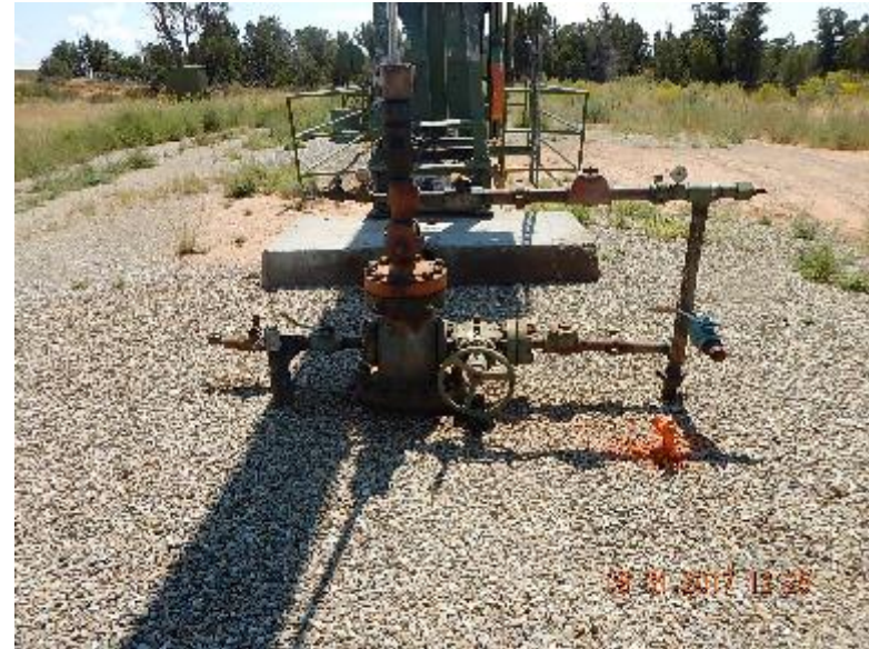
Photo 2: Wellhead and riser.
