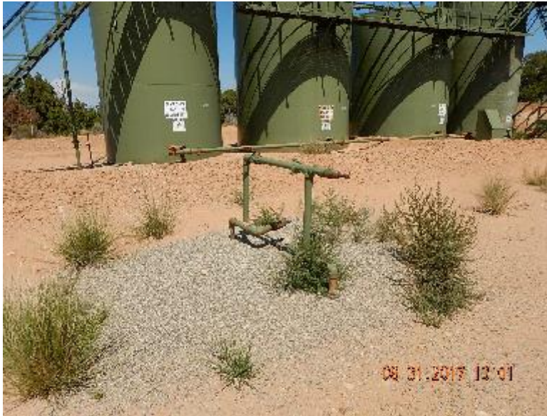
Photo 5: Riser outside of production tank berms.
