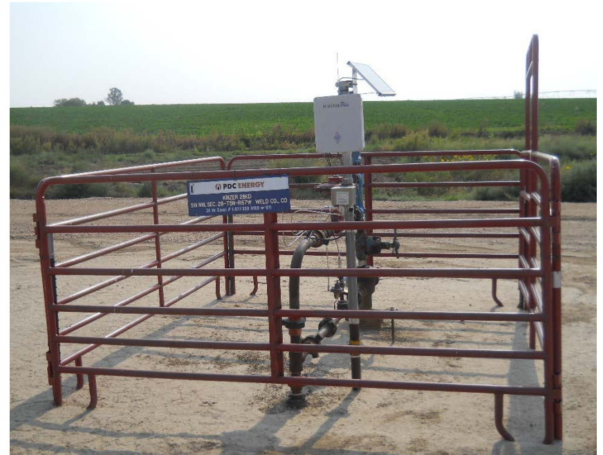
Kinzer 28KD wellhead looking east
