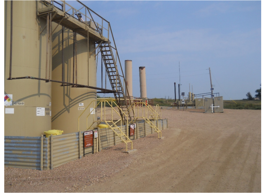
Battery looking northwest
