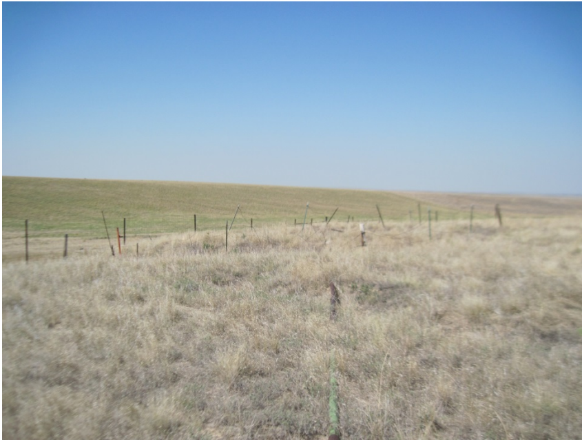
PIT FENCE IN DIS-REPAIR AND UNUSED PIPE
