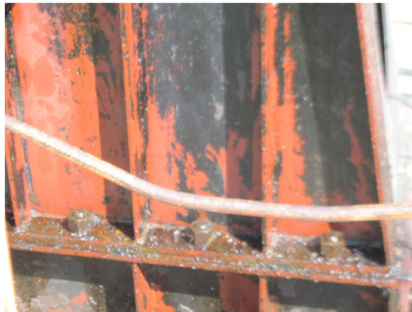
GEAR BOX LEAKING ON GROUND
