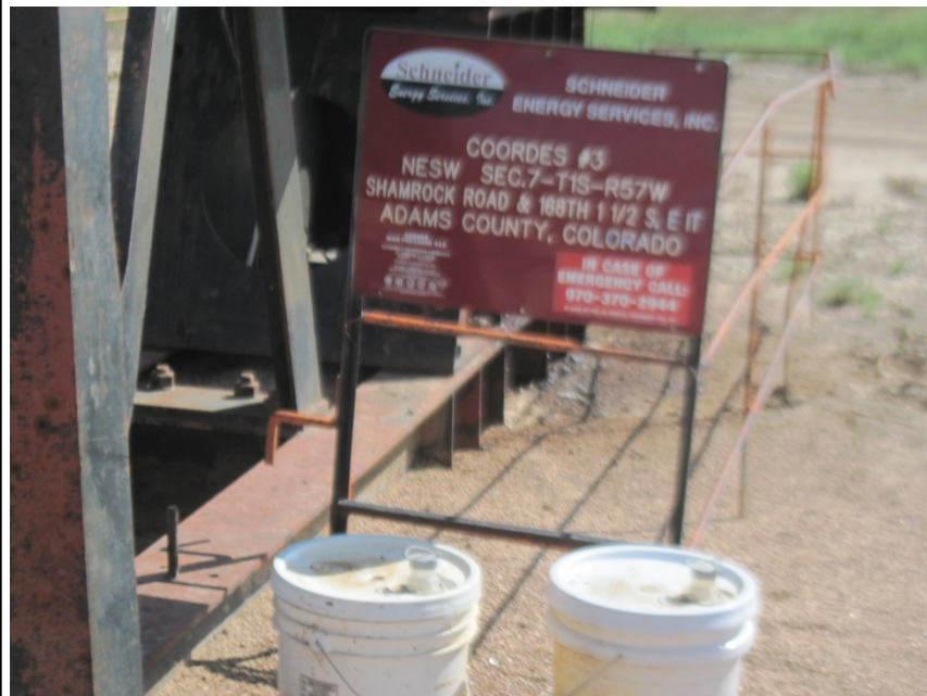
WELLHEAD, PUMP JACK AND TRASH
