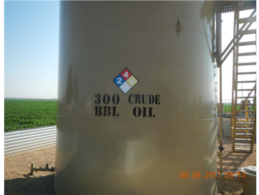
Crude oil tank placards
