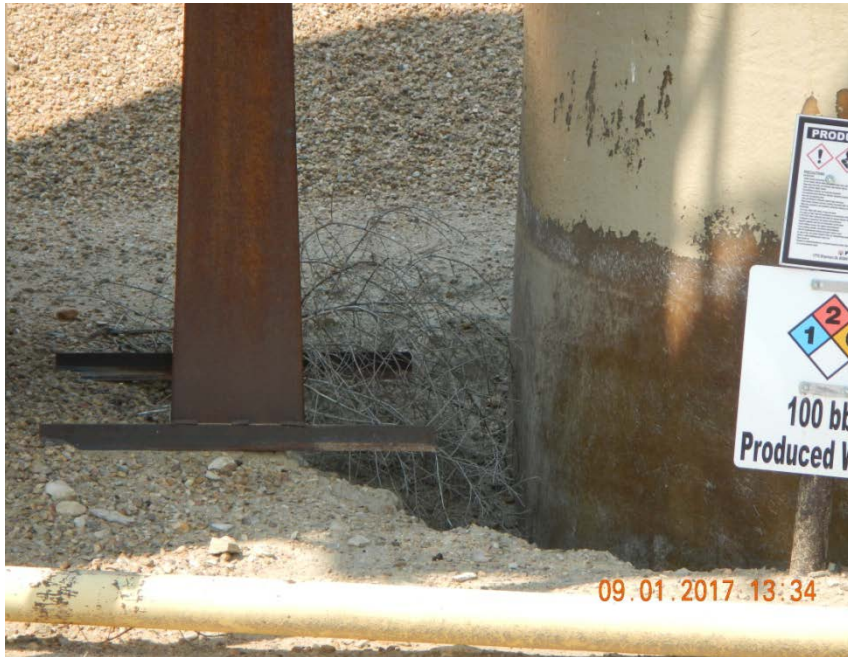
Produced water vault subsidence
