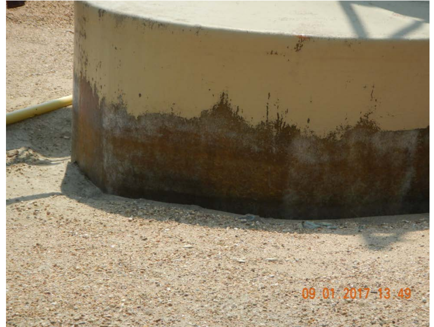
Produced water vault subsidence
