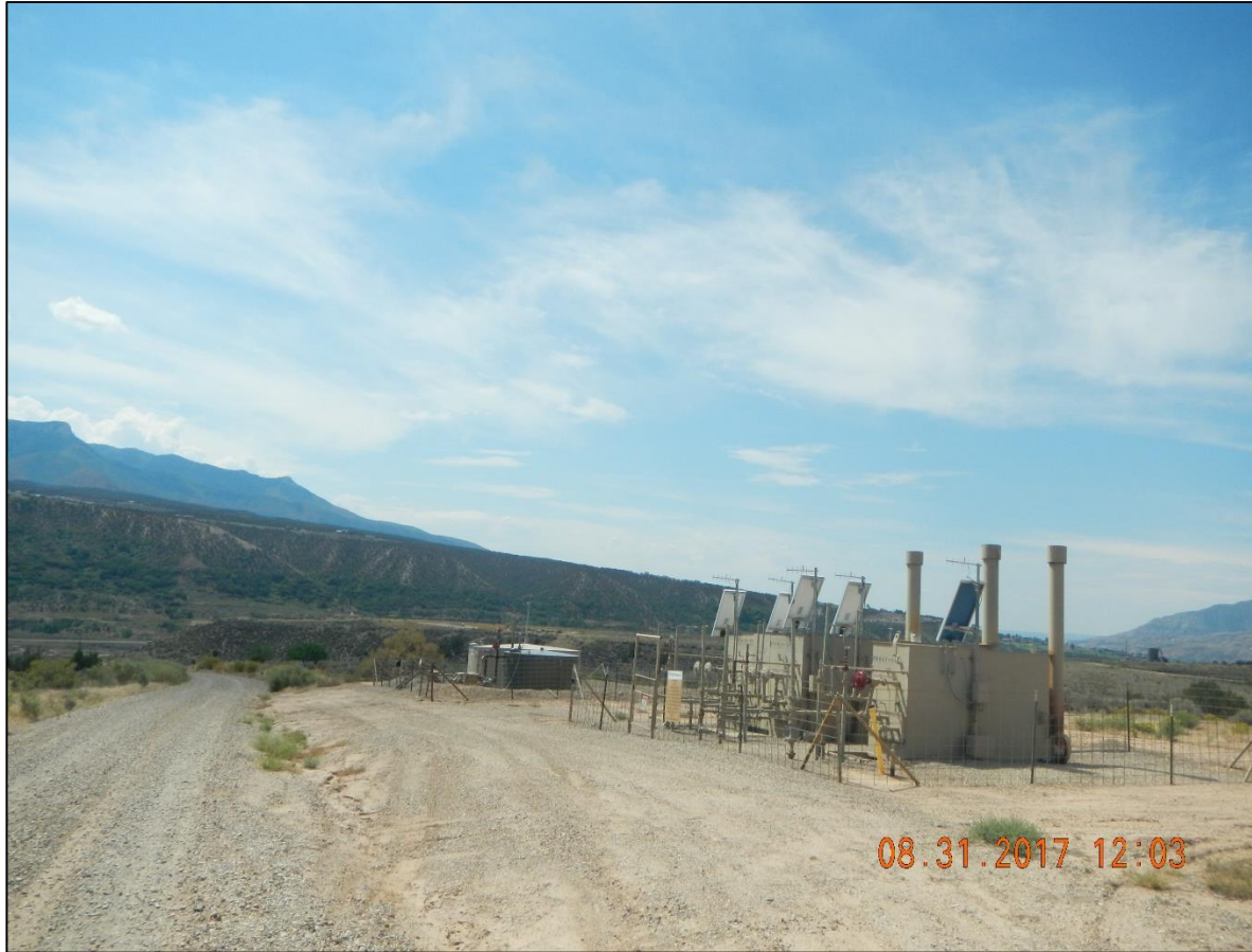
Separators and tank battery
