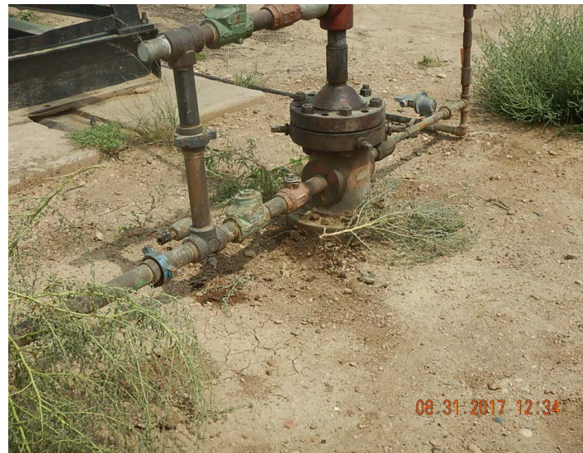
Photo 1: Trash removed, stained soil at wellhead.
