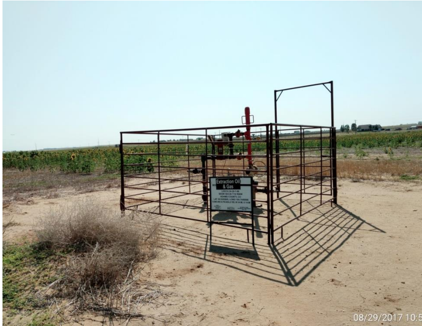
Wellhead Corrective Action: Signage missing emergency contact info.
