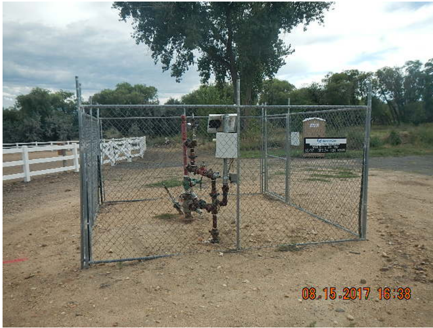
Well head taken from the North
