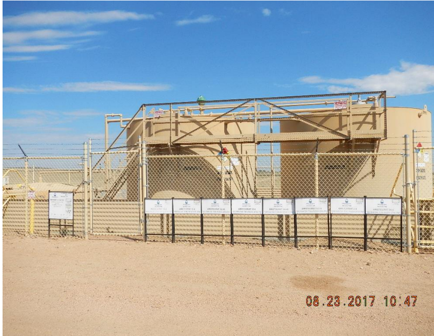
Photo 1: Battery from south
