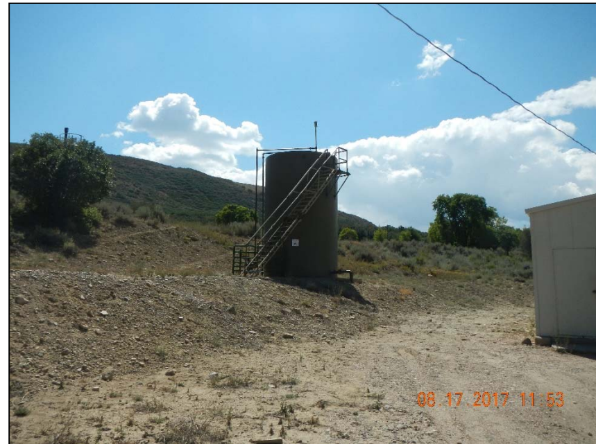
Photo 2. No berm around produced water tank.
