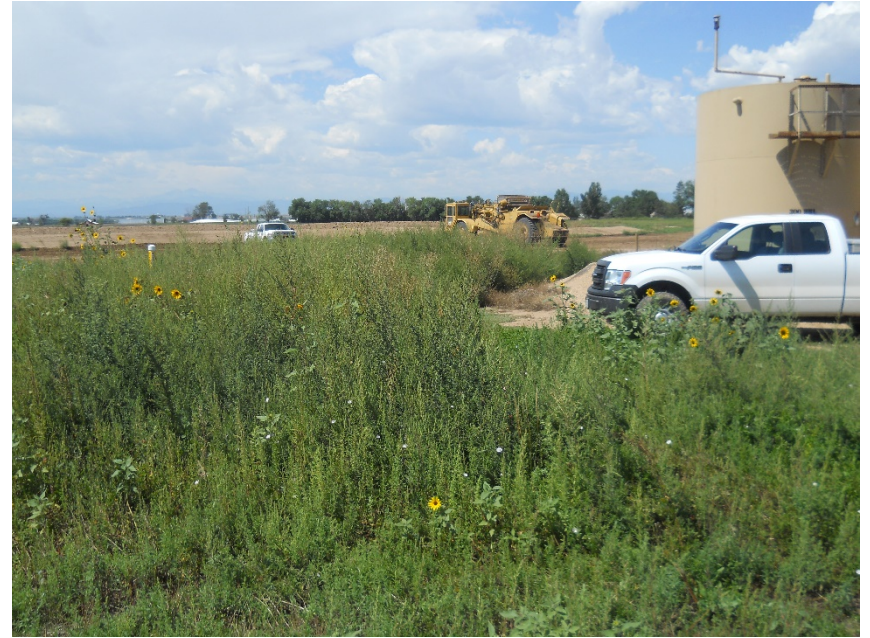
Actively growing weeds south perimeter of location looking west
