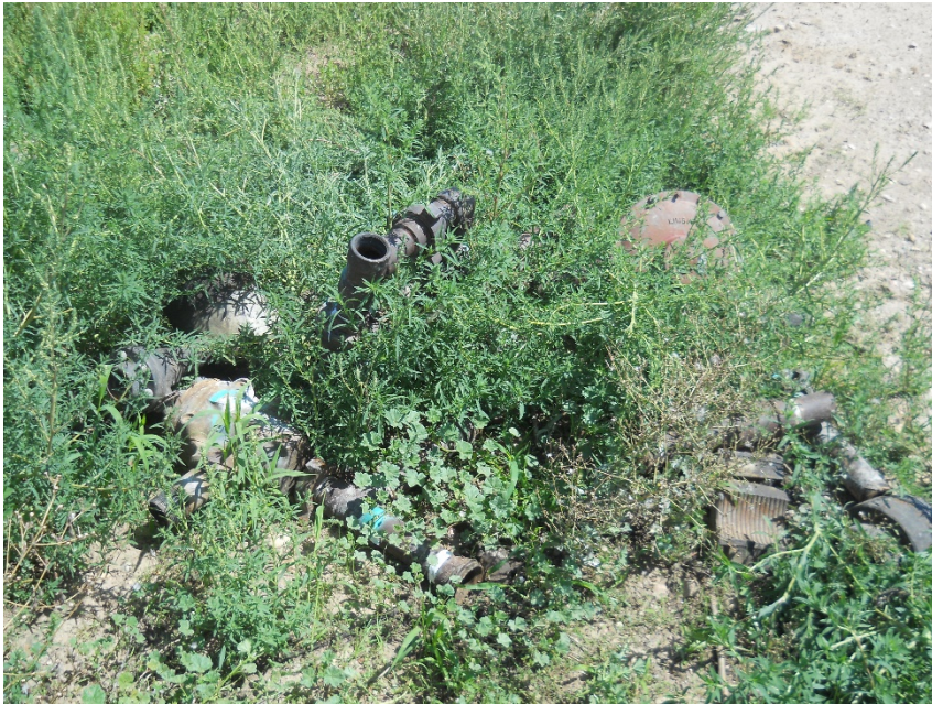
Wellhead equipment west edge of PA location
