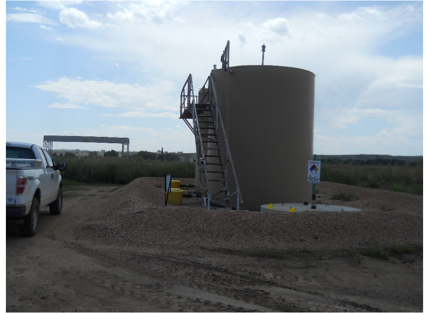
Tank battery looking south from separator
