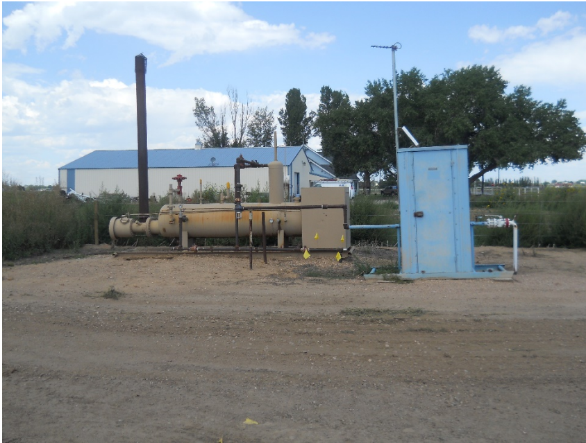
Separator and gas meter run looking north
