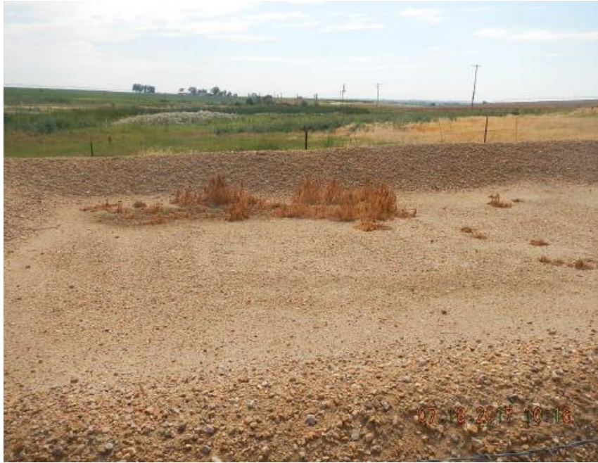
Photo 5: Previous inspection, weed debris within berm.
