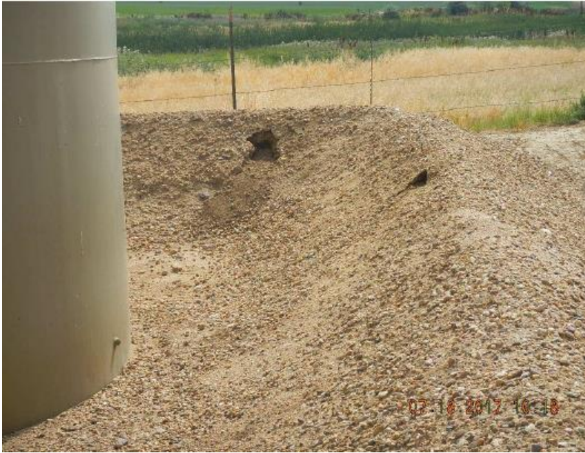
Photo 3: Previous inspection, compromised berm
