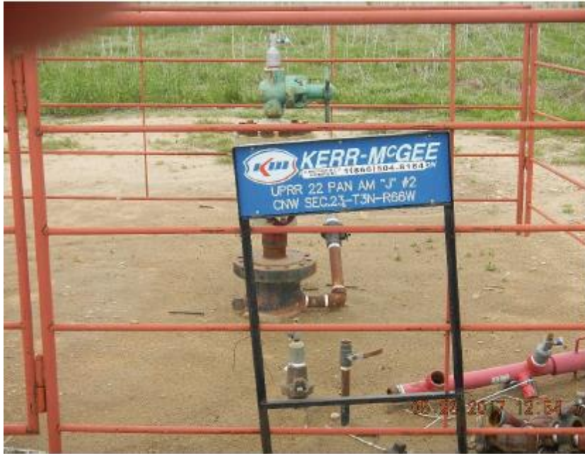
Photo 1: Unused equipment at wellhead from previous inspection.
