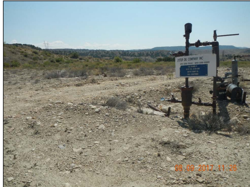
Photo 2. Debris at wellhead.
