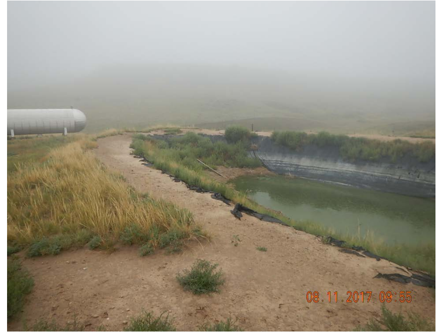
Photo 2: Pit liner sagging
