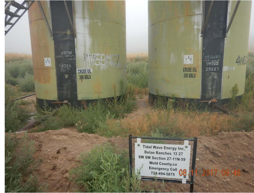
Photo 5: Tanks have placarding, contents, capacities. Operator signage and emergency number at battery. Weeds in berms
