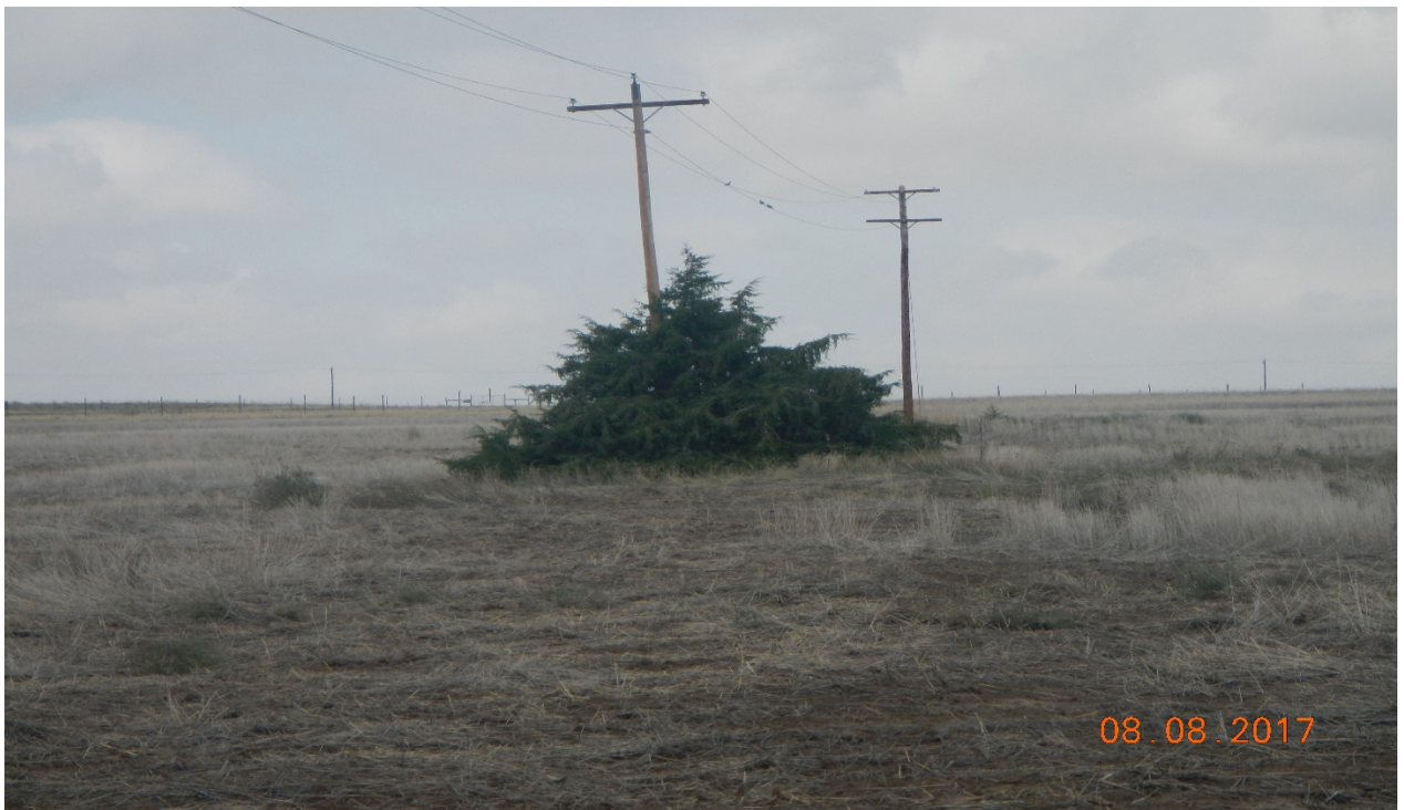
photo 2: The electric utility line terminates at the location.
